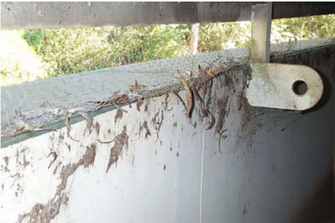
Figure 8: Ventilation mesh not effective against leaf debris and wind born contamination.
