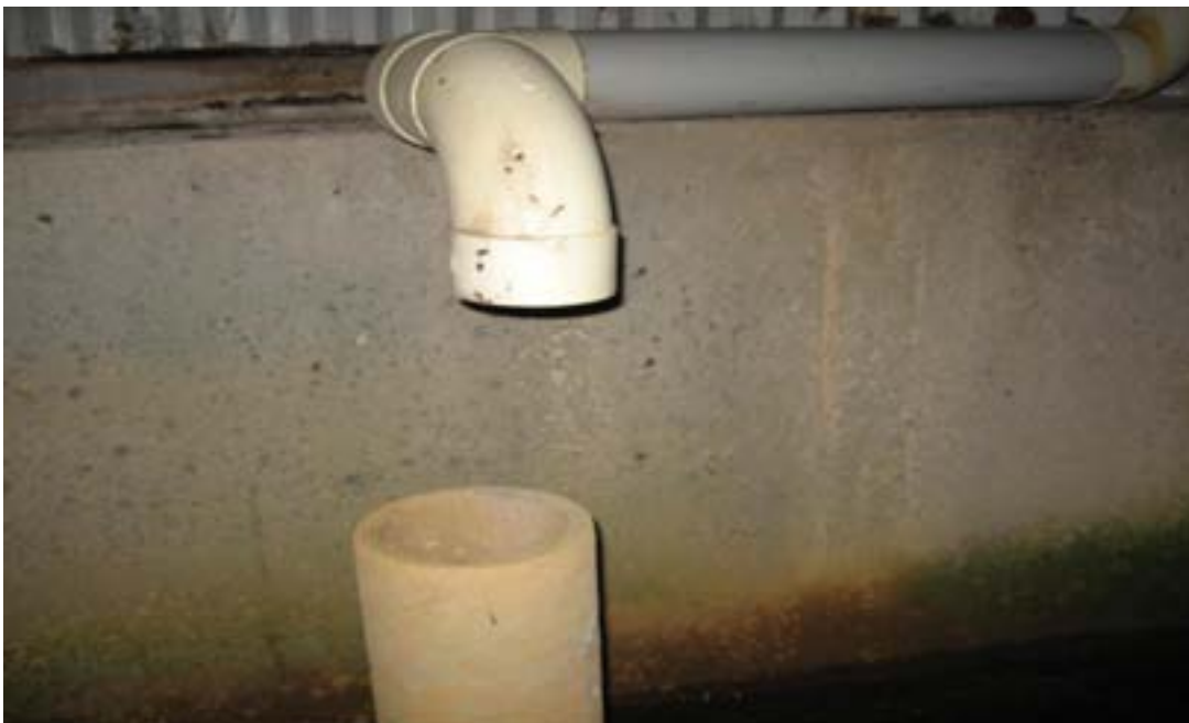
Figure 7: A roof drain point not connected into the overflow.
