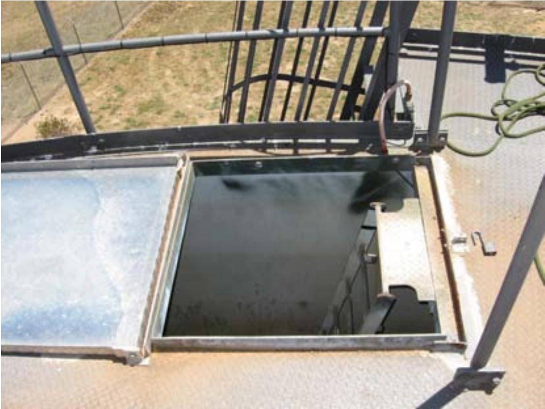
Figure 4: The existing ladder stiles trimmed off, the front edge sealed and an overlapping cover fitted.
