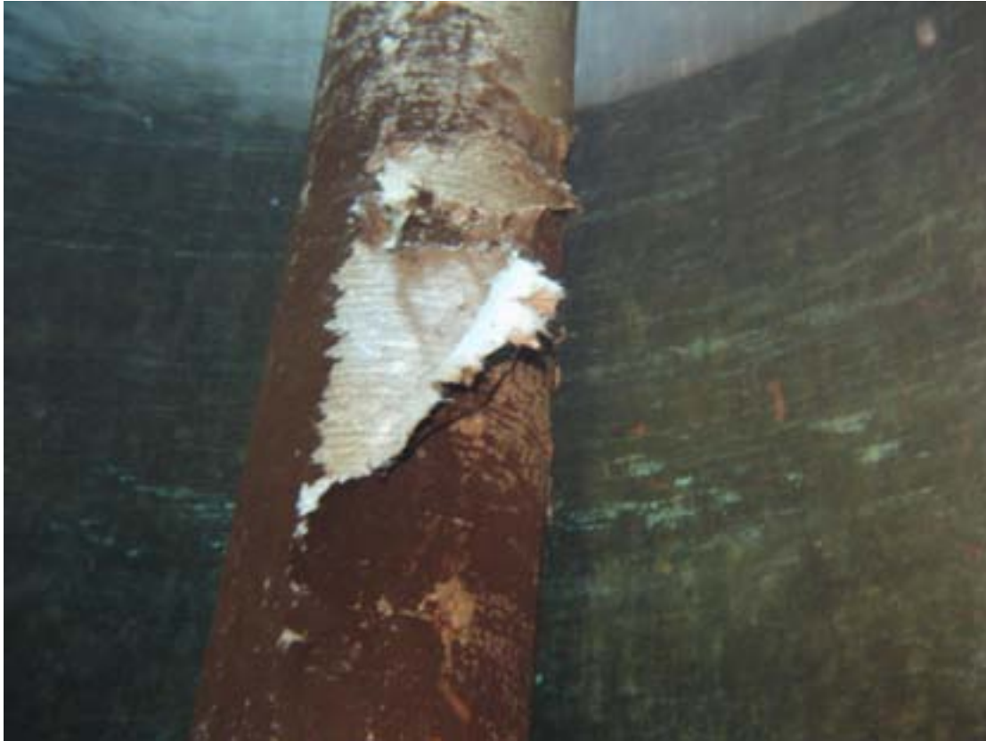
Figure 9: An AC overflow riser pipe that is de-laminating.
