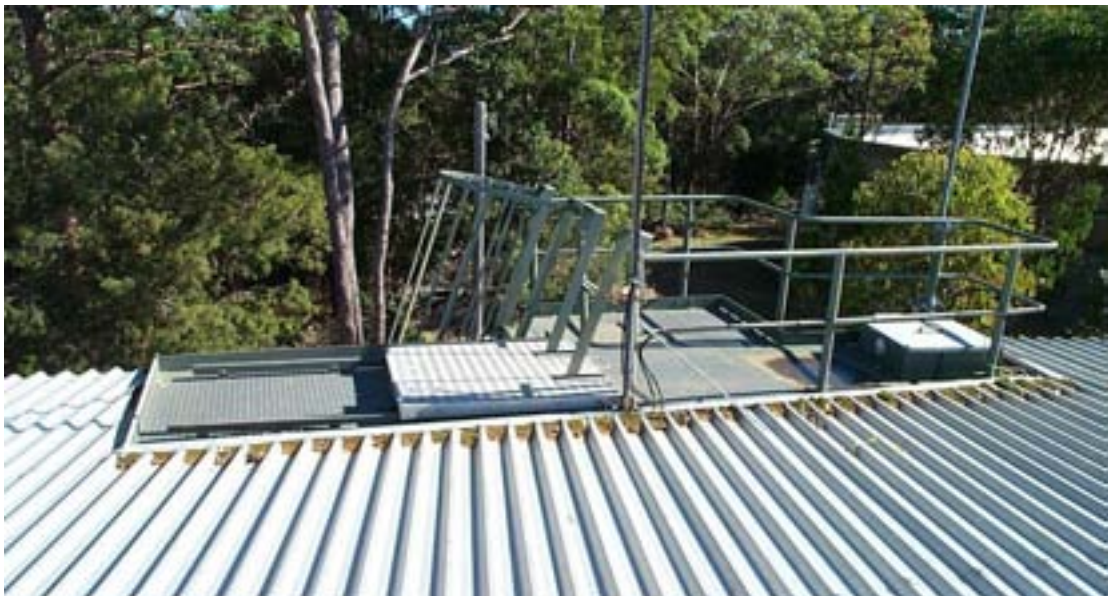
Figure 5: Typical platform area – roof debris is ponding, unsealed hatch area and lack of effective guard rails.
