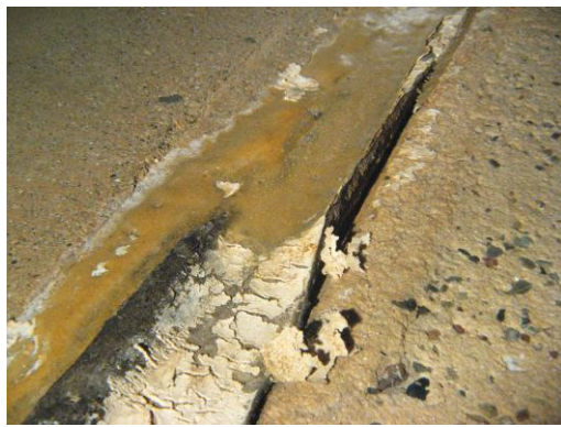
Figure 17 Subsided floor seal
