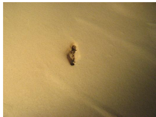
Figure 18 Floor leak indicated by absence of sediment
